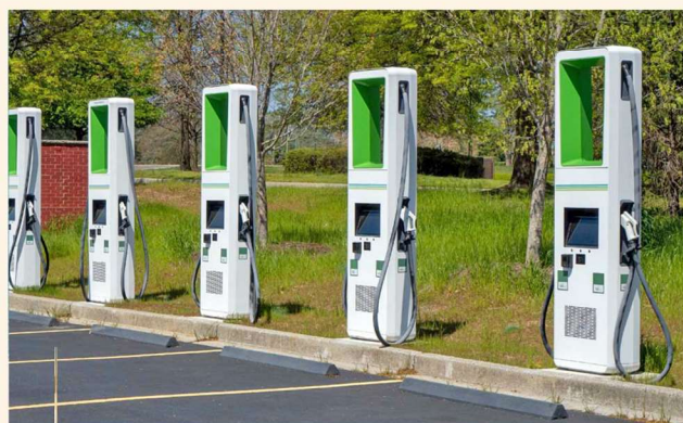
O5. EV CHARGING STATION
